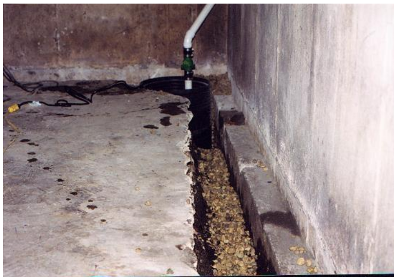
Figure 1 – Interior Foundation Drainage System with Sump Pump
